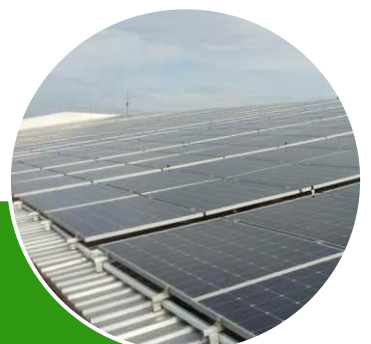
Ajantha Polymer 100 KW, On Grid Systems, Sangari
