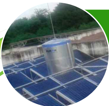
Erode Sengunthar Engineering College 6000 Litre, Perundurai
