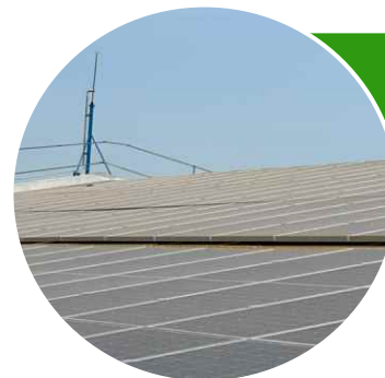
Gemrose Spinning Mills 500 KW Solar Grid System, Annur
