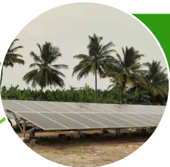
Perundurai Village Panchayat Solar Water Pumping System 35 KW Water Pumping System
